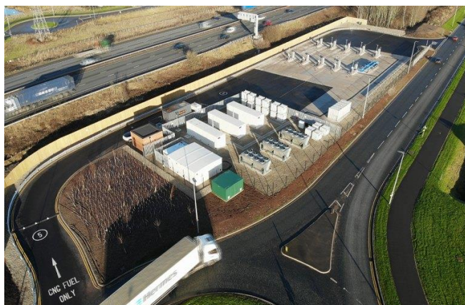
Figure 7: Warrington bio-CNG refuelling station
