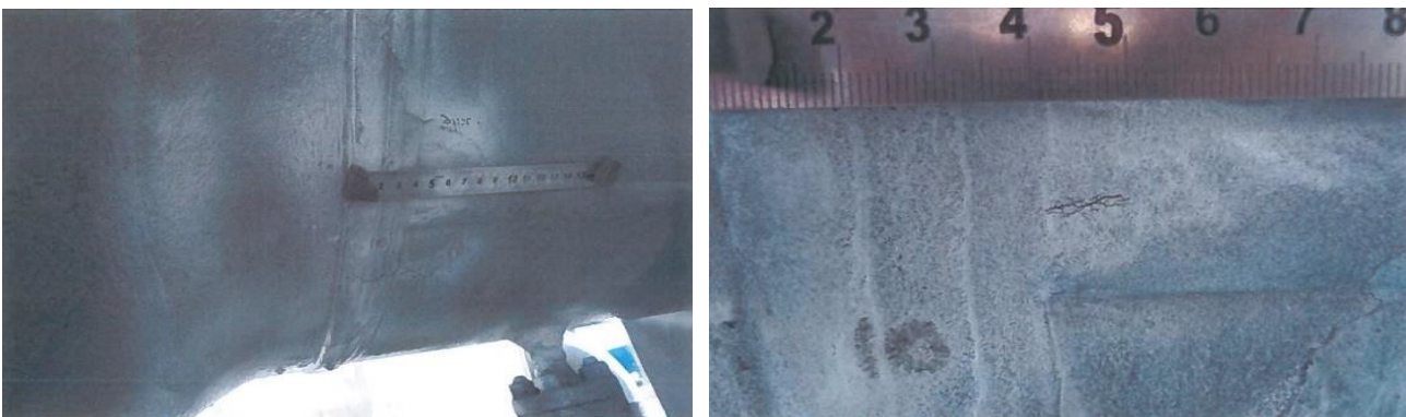
A 10mm crater crack in a longitudinal sub arc weld to the front end of a filter.
