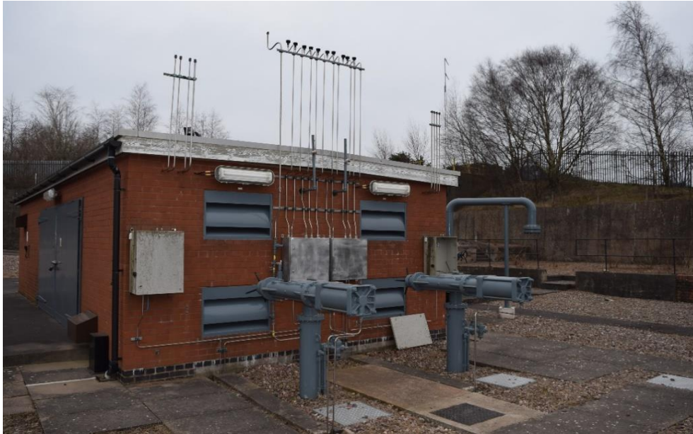
Figure 1: Pressure-Regulating installation showing filters in the foreground, monitors and vented building behind
